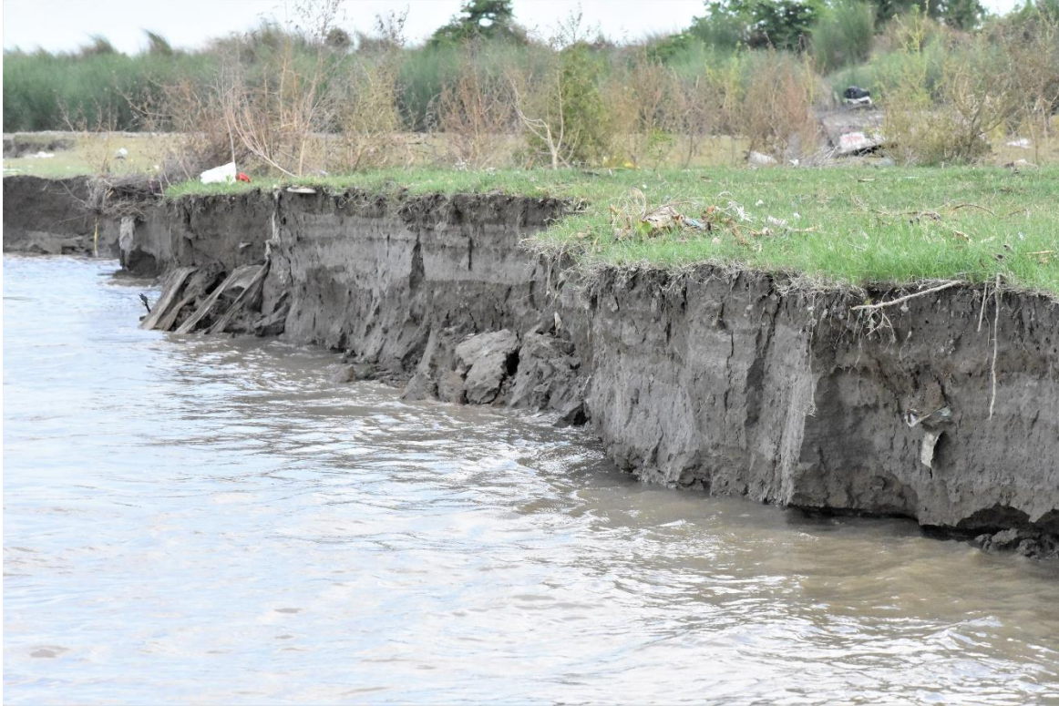
Image 42 : Erosion Prone Bank As Observed Below Mehendipur Ghat Bridge
